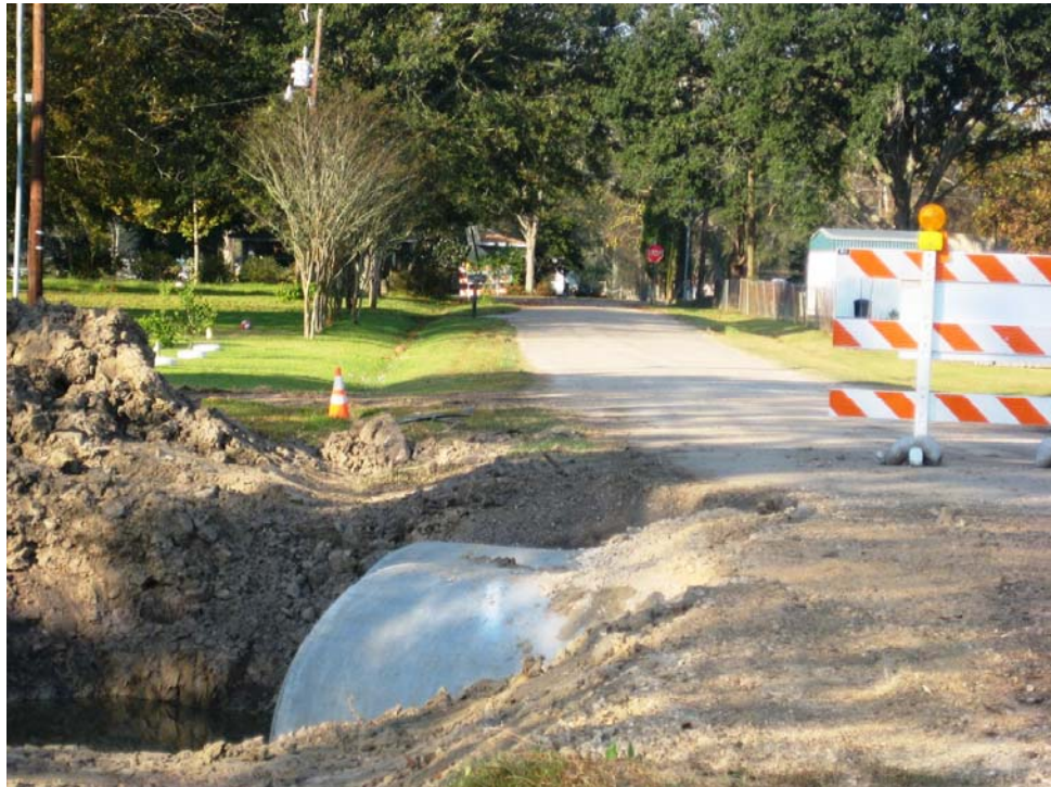
George.Duplessis.111609.2 – Work continues in this Nov. 16 photo to replace a wooden bridge on George Duplessis Road with several large 60-inch concrete culverts as seen here.
