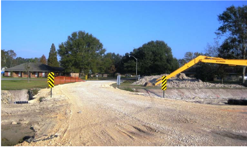
George.Duplessis.111609.1 – Local motorists are advised to use this temporary connection with Betty Street during ongoing construction on George Duplessis Road.
